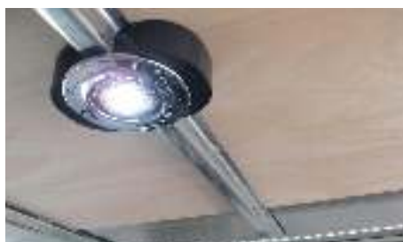
Advanced Lighting Package
